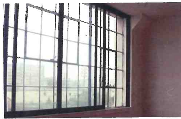
Recommended Original metal windows were retained and made operable during the rehabilitation of this historic mill complex. Installing patio slider doors as interior storm windows was a creative and successful solution to improve the energy efficiency of the existing windows.
