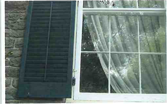
Recommended Historic exterior storm windows have been well maintained and continue to perform as intended.
