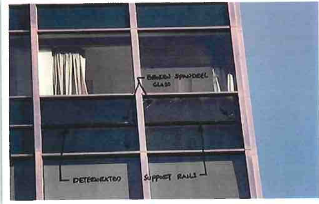
Recommended The original windows, which were deteriorated beyond repair, featured a dark tint. They were replaced with a slightly lighter-tinted glazing to improve daylighting in this mid-century modern office building.
