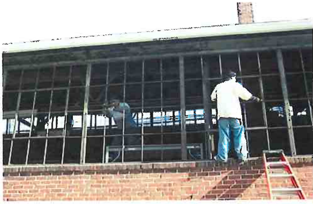
Recommended Original metal windows were appropriately repaired as part of the rehabilitation of this historic industrial building. During rehabilitation.
