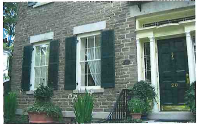
Recommended Historic exterior storm windows have been well maintained and continue to perform as intended.
