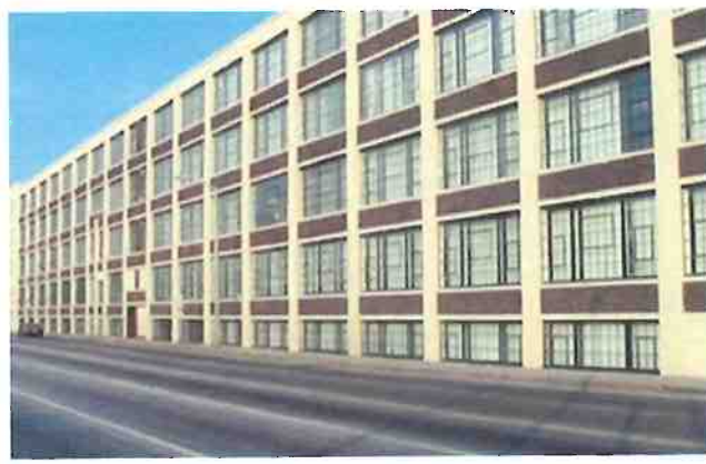
Recommended Original metal windows were retained and made operable during the rehabilitation of this historic mill complex. Installing patio slider doors as interior storm windows was a creative and successful solution to improve the energy efficiency of the existing windows.
