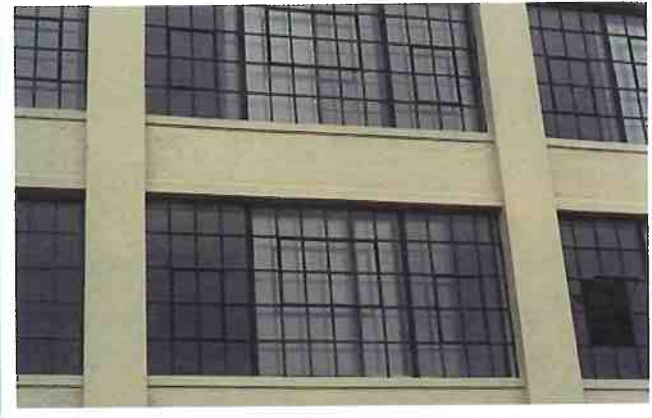
Recommended Original metal windows were retained and made operable during the rehabilitation of this historic mill complex. Installing patio slider doors as interior storm windows was a creative and successful solution to improve the energy efficiency of the existing windows.
