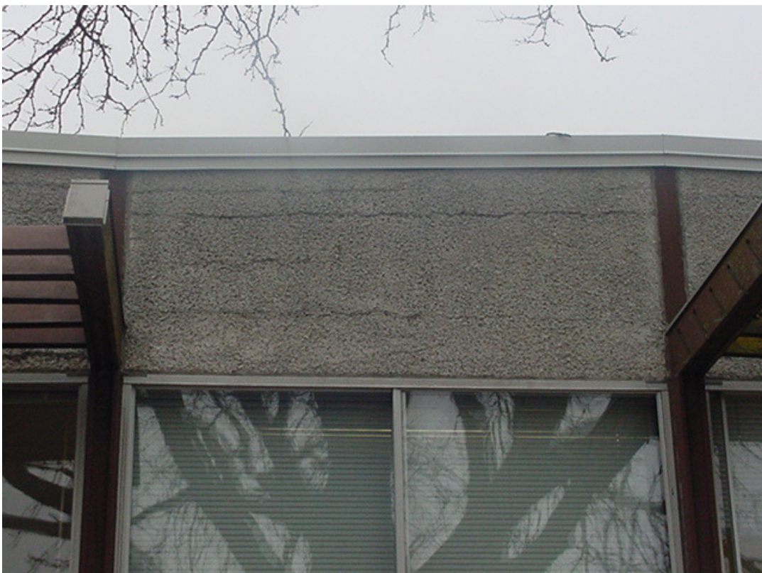
No. 8 Existing South (Front) Stucco: Deteriorating stucco bulging and cracking to be fully removed and replaced with EFIS.
