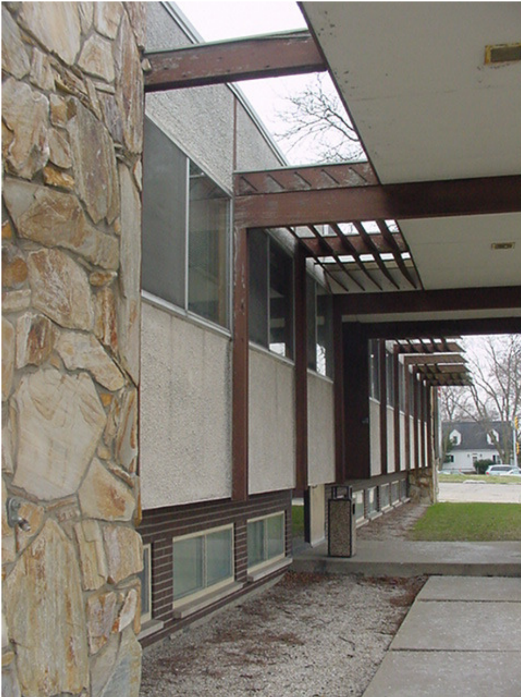
No. 3: Existing South Elevation (Looking East): Sun Shades to Be Removed and Vertical Wood columns between Windows to be Removed; all deteriorating stucco to be removed and replace with EFIS; Windows to be replaced with bronze frames, tinted windows.
