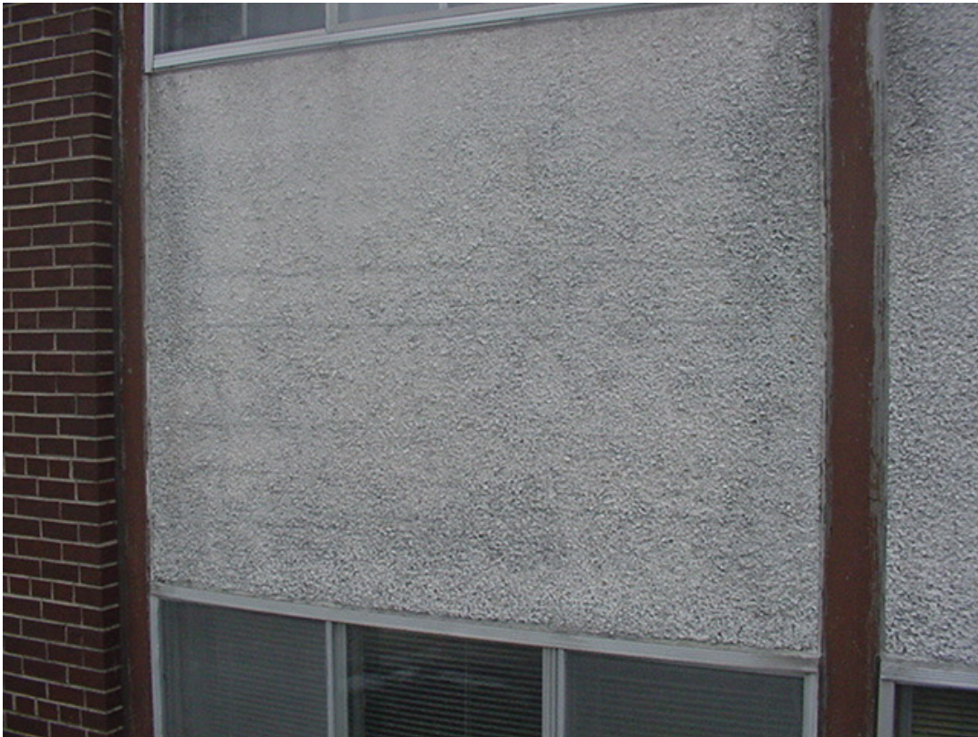
No. 15 Existing North (Back) Stucco: Deteriorating stucco bulging and cracking to be fully removed and replaced with EFIS.
