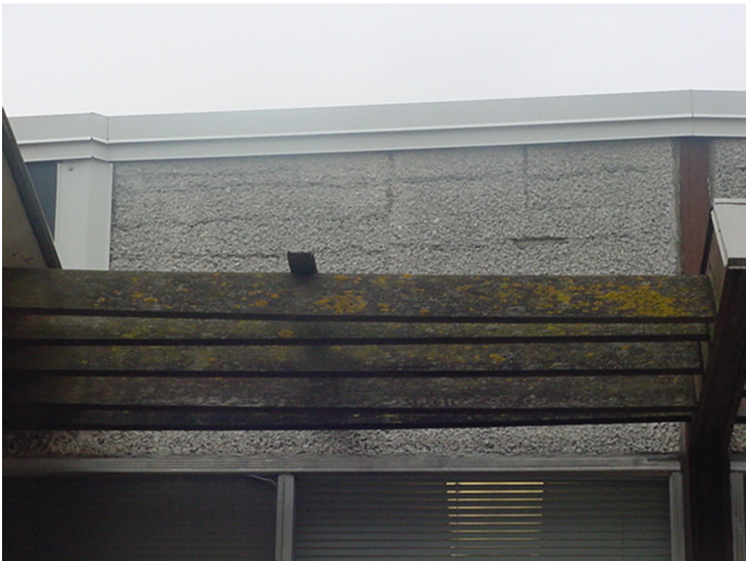
No. 6 Existing South (Front) Stucco: Deteriorating stucco bulging and cracking to be removed and replaced with EIFS.
