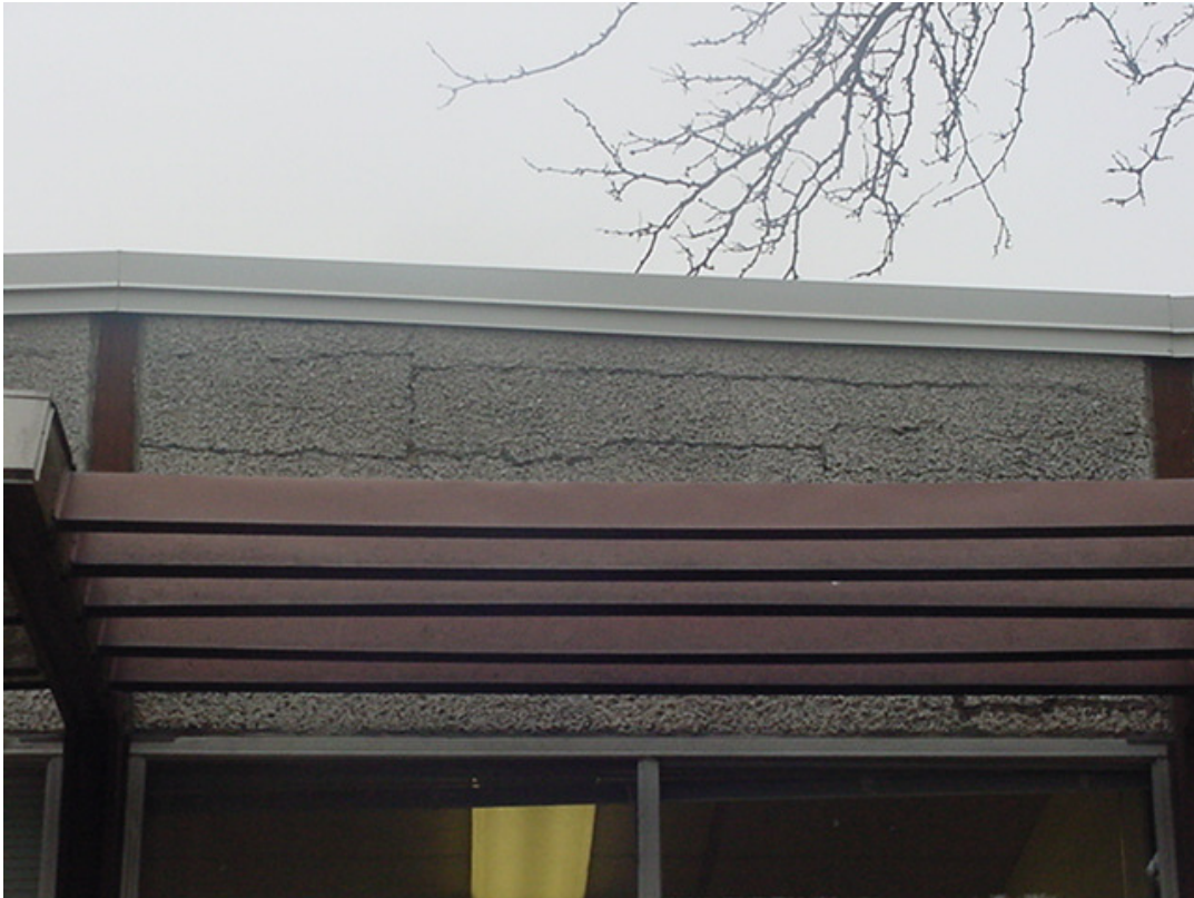
No. 7 Existing South (Front) Stucco: Deteriorating stucco bulging and cracking to be fully removed and replaced with EFIS.
