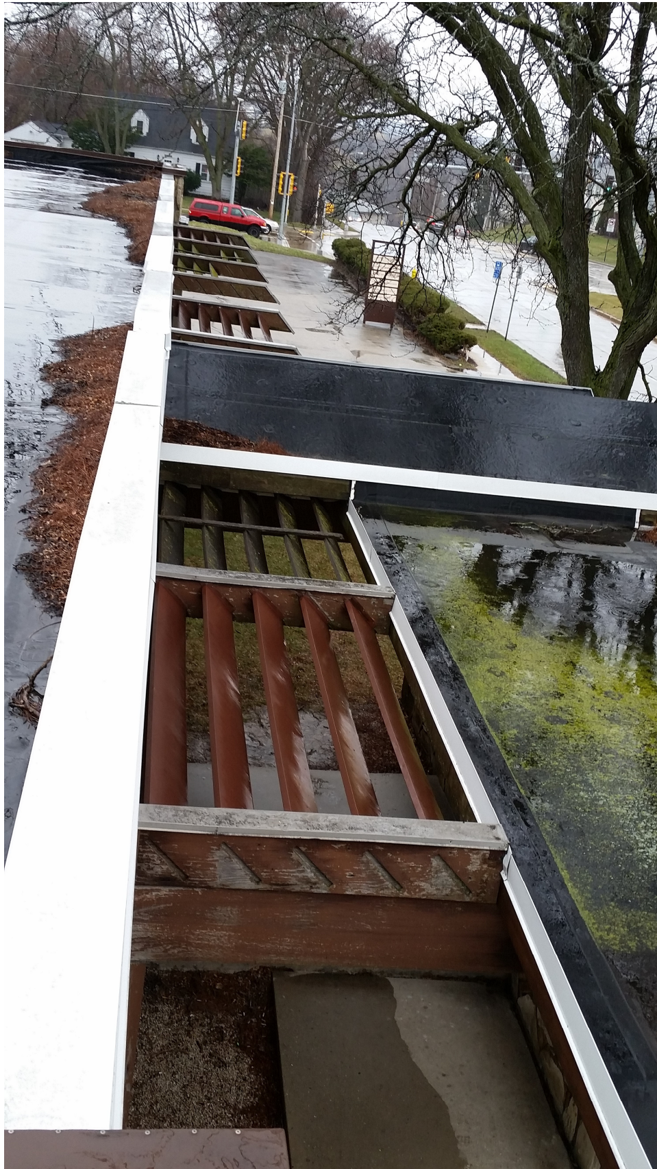
No. 4: Existing South (Front) Sun Shades: Roof View of the Sun Shades beams and wood boards that are to Be Removed.
