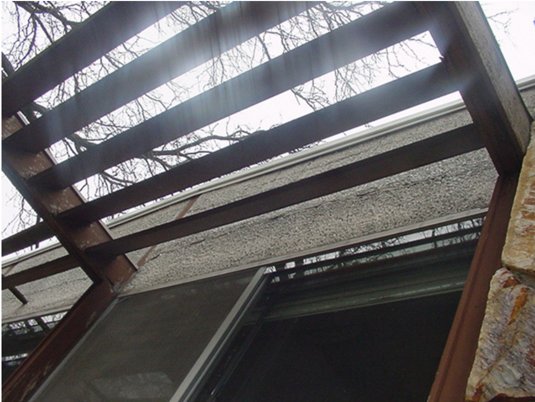
No. 5 Existing South (Front) Stucco: deteriorating stucco bulging and cracking to be removed and replaced with EIFS.
