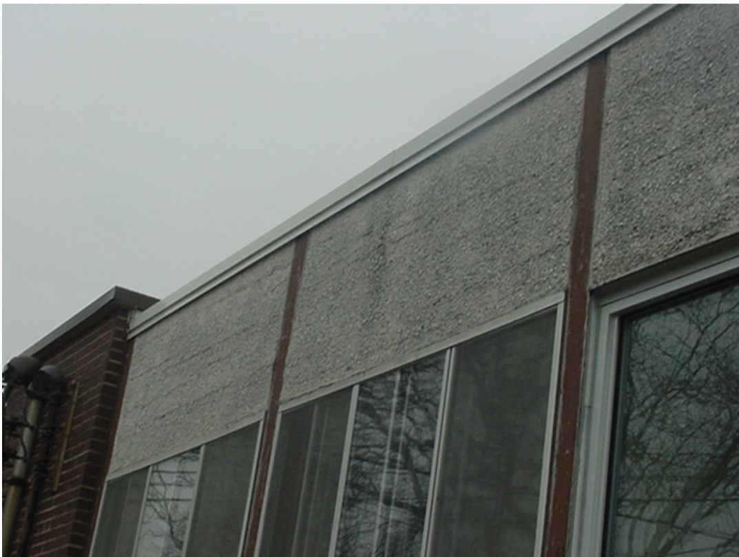
No. 14 Existing North (Back) Stucco: Deteriorating stucco bulging and cracking to be fully removed and replaced with EFIS.
