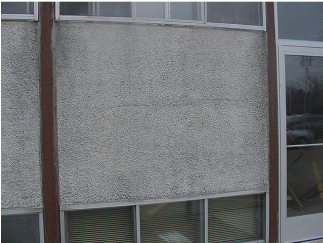
No. 16 Existing North (Back) Stucco: Deteriorating stucco bulging and cracking to be fully removed and replaced with EFIS.
