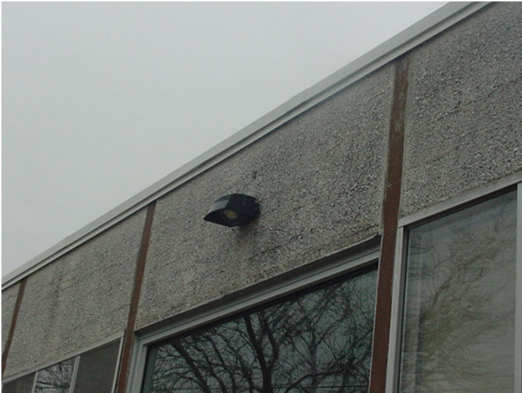
No. 13 Existing North (Back) Stucco: Deteriorating stucco bulging and cracking to be fully removed and replaced with EFIS.
