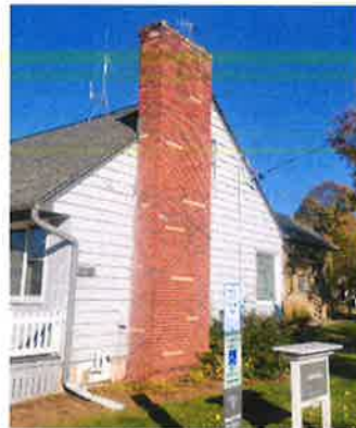
South Elevation: Carroll University Public Safety House. Chimney will be restored to match original construction.
