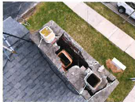
Chimney Top: Carroll University Public Safety House. Cap to be restored with dummy flues.
