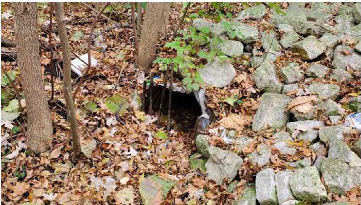
This is a picture standing near Wetland 1 facing the culvert which drains into the wetland.
