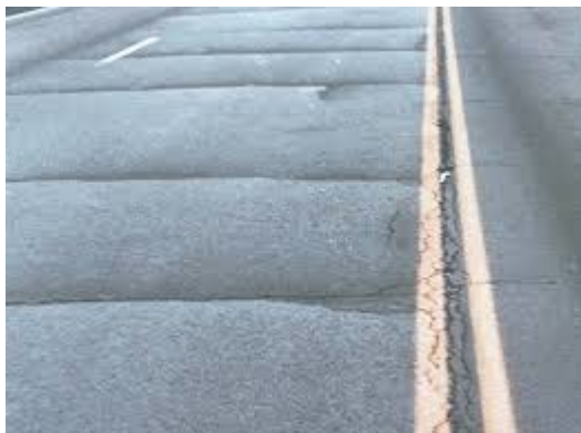
Block Cracking - Medium
