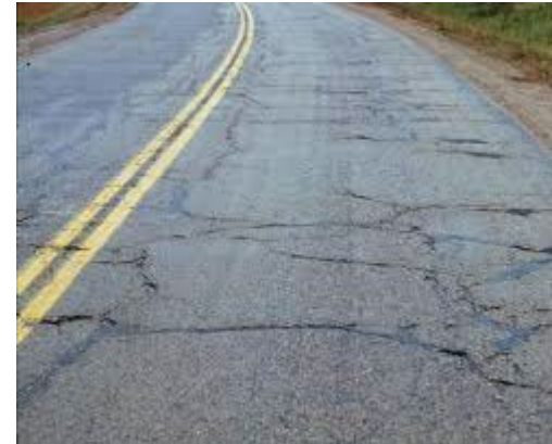
Block Cracking - High
