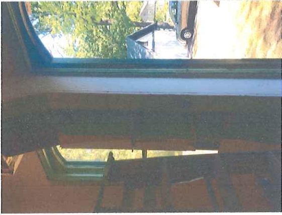
exposed beams supporting chimney... end at kitchen floor (not in basement)
