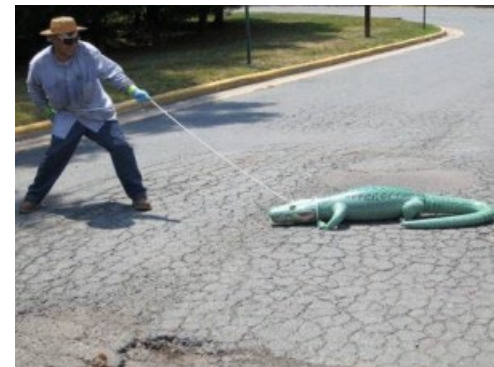
Alligator Cracking (Leads to potholes)
