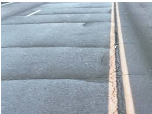
Block Cracking - Medium
