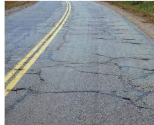
Block Cracking - High
