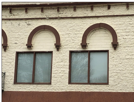
Replacement windows that do not match the original size and style can damage your building's historic integrity.
