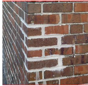
Mortar that does not match existing can damage historic character and surrounding masonry. (Photo Credit: Wisconsin Historical Society)
