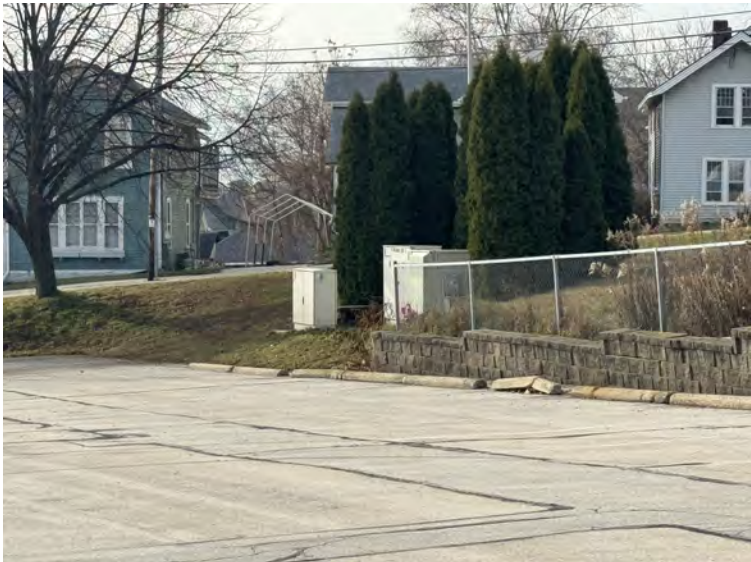
Photograph 6 - Transformers on 130 Delafield St
