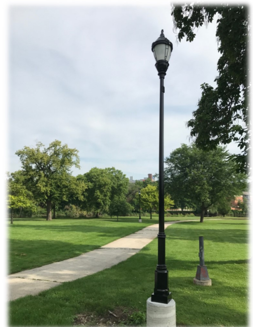
New LED lights installed at Bethesda Park
