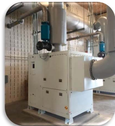
Use of efficient high-speed turbo blowers in place of the existing 700 hp and 350 hp aeration blowers will provide a significant energy reduction for the plant.
