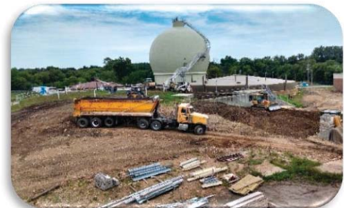
An egg-shaped digester was chosen over traditional technologies, as it alleviated solids deposition, improved processes, and provided operational benefits.
