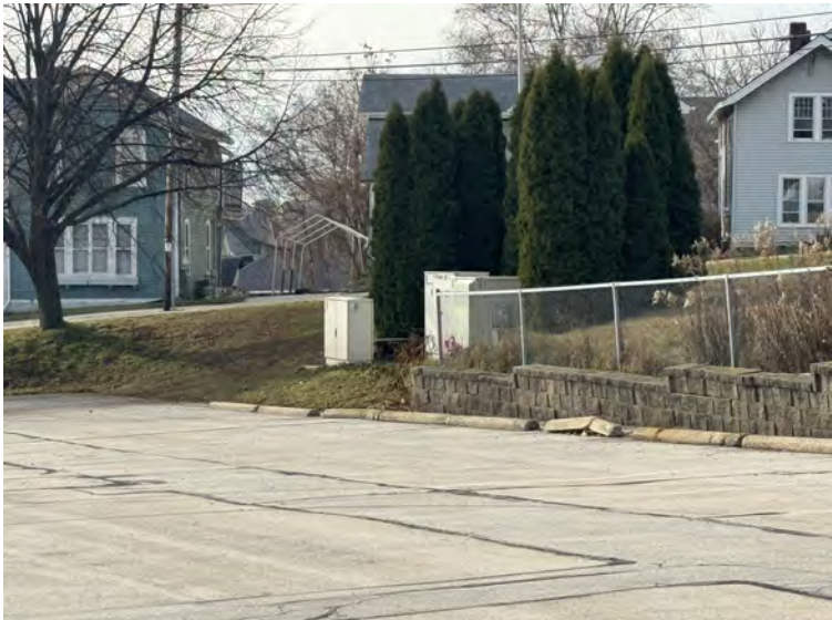
Photograph 6 - Transformers on 130 Delafield St
