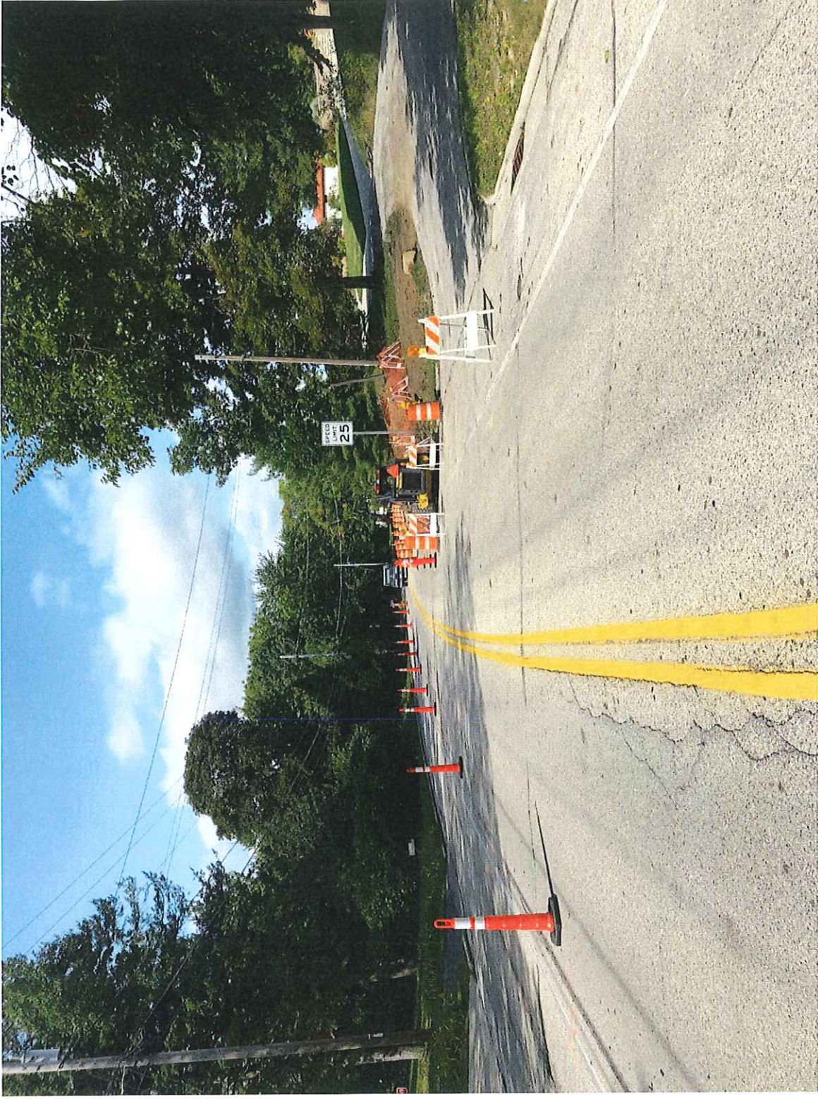
East end of the beginning of the work zone looking East. Following the accident(s), the skid loader was moved to this end to better protect and highlight the work area.
