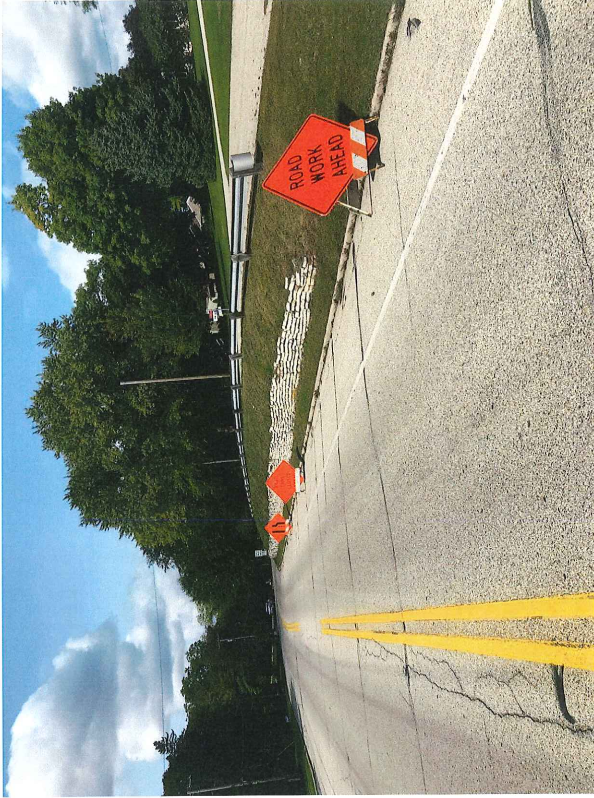
Work Ahead signs on Broadway, approximately 600 feet East of the work zone.
