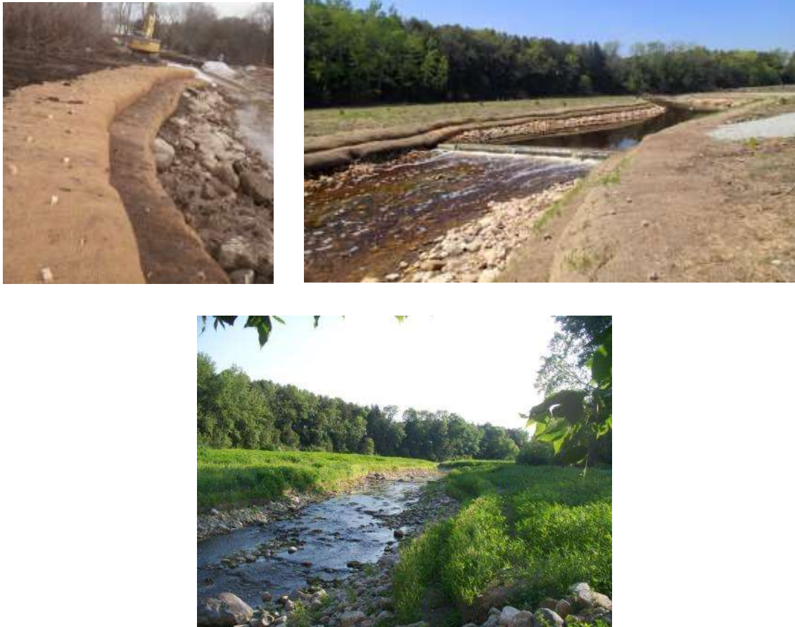
Figure 9. Construction and Post-Construction Photos of Bank Stabilization in Former Impoundment of Bruemmerville Dam, Algoma WI (Courtesy of Cardno Inc. and Kewaunee County)
