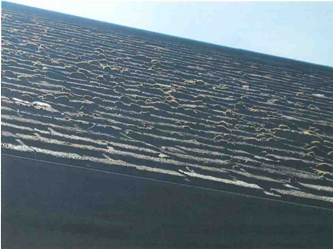
Moss growing on roof
