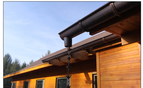
A detail view of the rainwater harvesting system.
