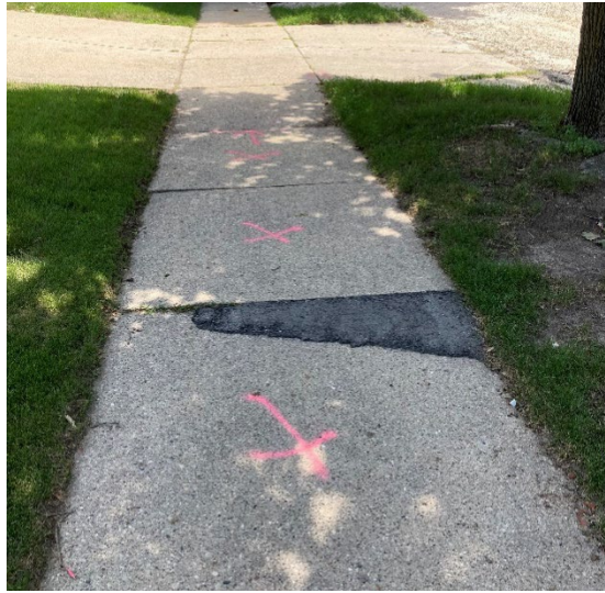
Figure 2: Tree Damaged Sidewalk Example
