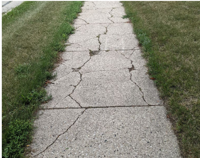
Figure 1: Condemned Criteria Sidewalk (Cracked with Pieces Missing)
