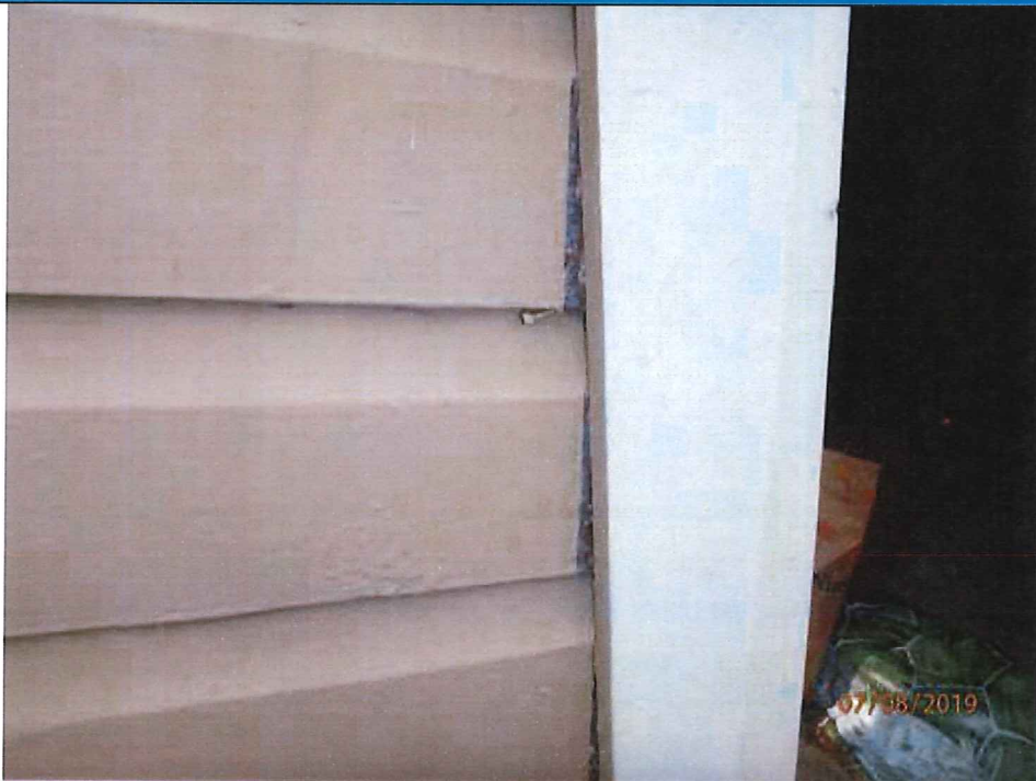
Photo 14: Exposed unpainted surfaces.
