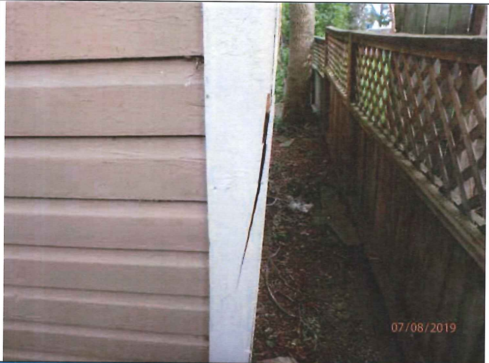
Photo 11: Fractured corner trim.
