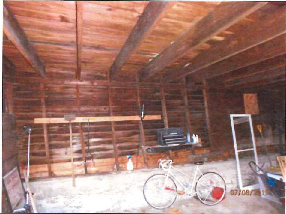
Photo 15: South wall of garage displaced to the east.
