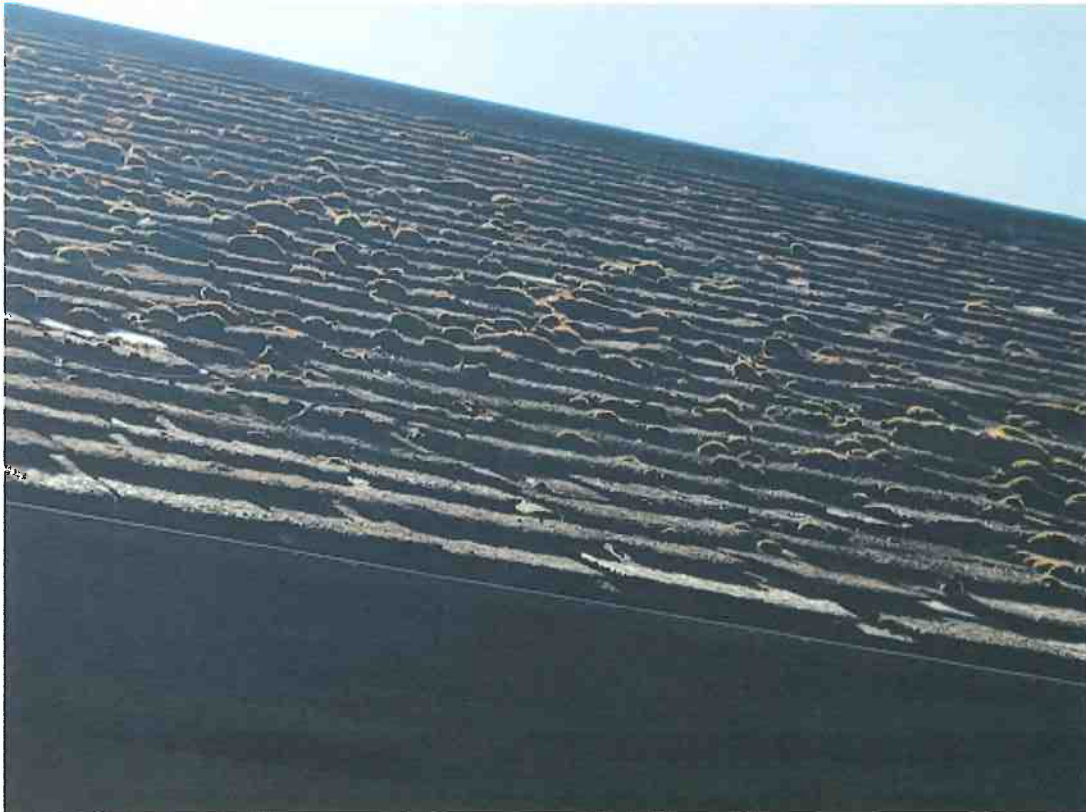
Moss growing on roof
