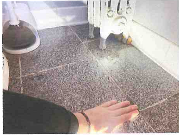
Half bathroom tiling not properly installed & unlevel
