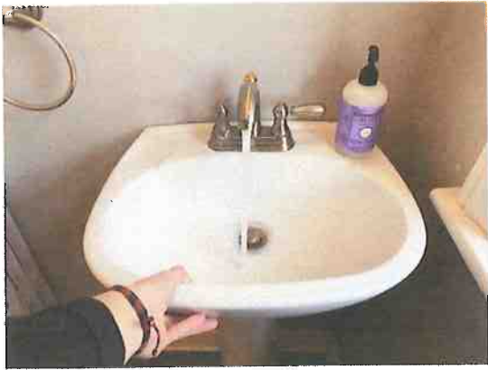
Half bathroom vanity loose & not level
