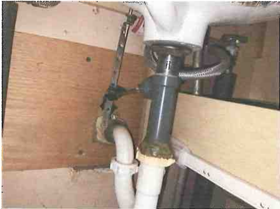
Improper repairs master bathroom sink
