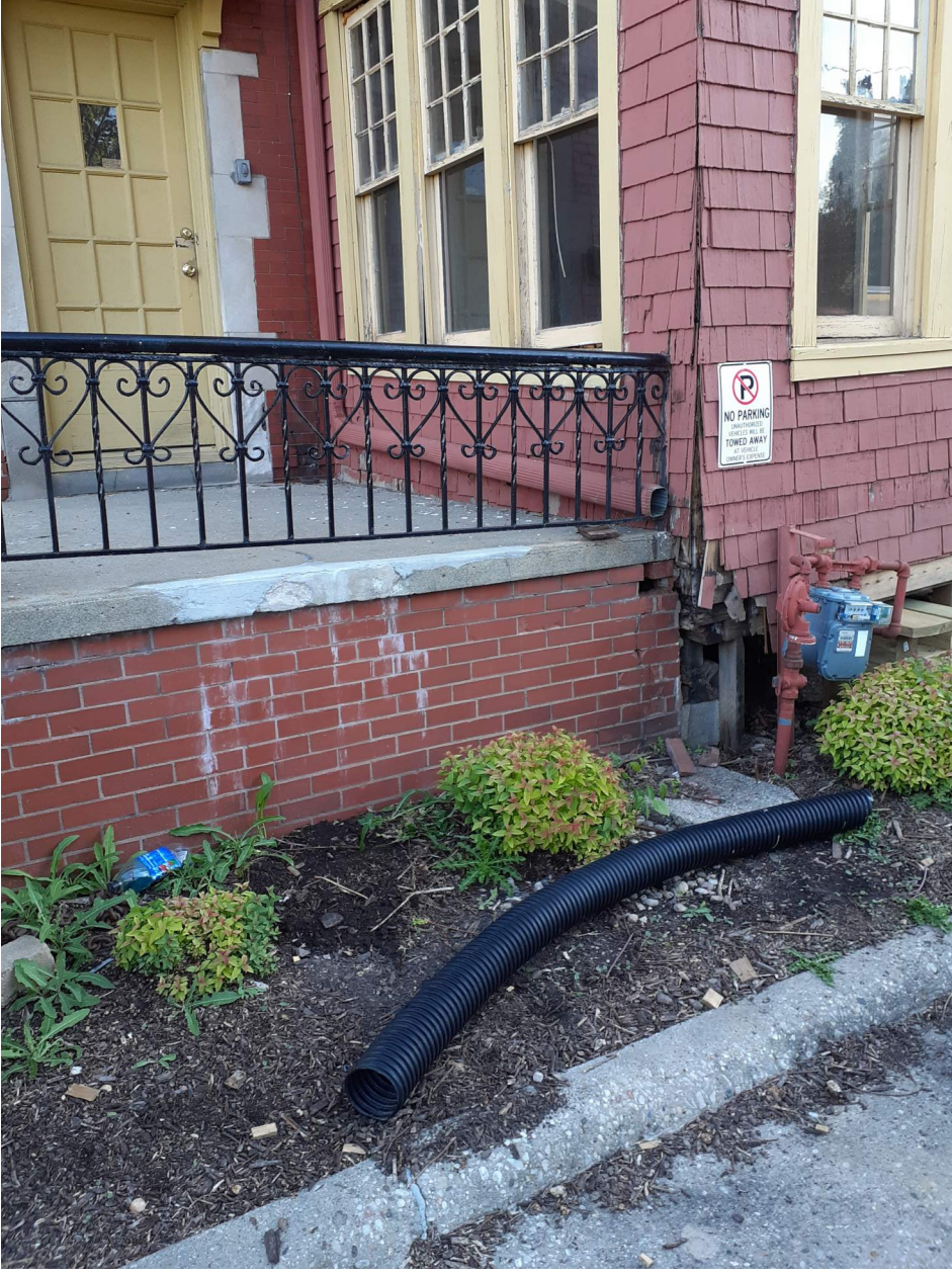
SINKING FOUNDATION @ GAS METER
